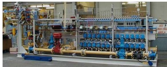
Gas valve skid fully assembled
