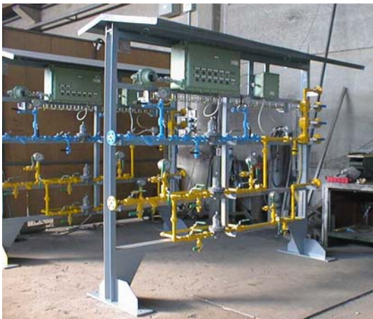
Flame front Generator Ignition Panel
